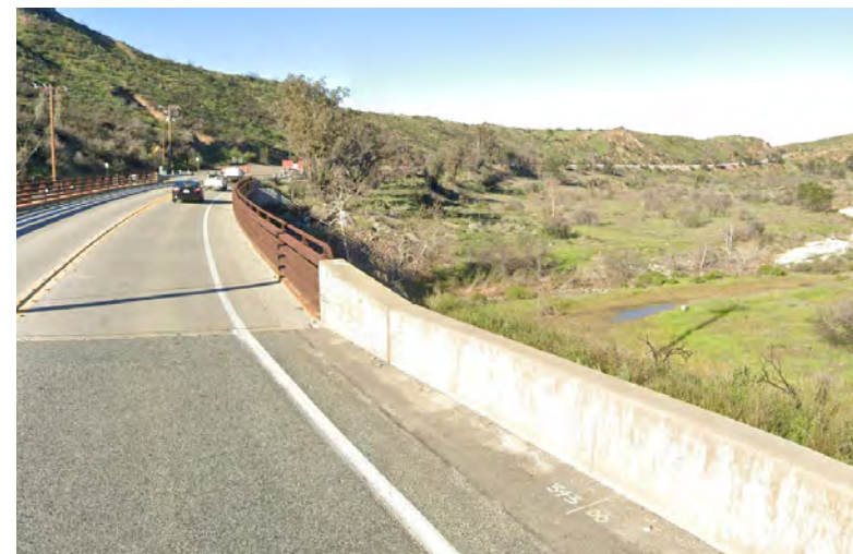
The recommended shared-use path will need to include bridges to navigate difficult areas like at this stream
