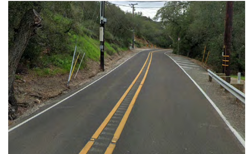
Utilities and forested areas will make paving the shoulder difficult in some areas of the street
